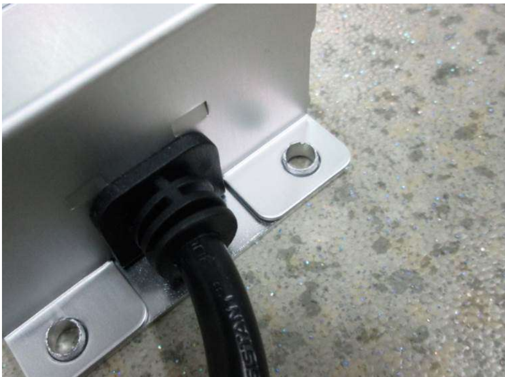
Earthing connection-1, ELG-100-54B
